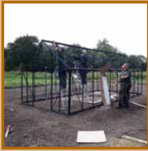
Sculthorpe volunteers building the greenhouse which will be the centre of the new community garden.
